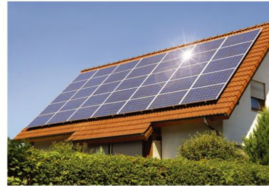
▲ Figure 12 A domestic photovoltaic panel system.
